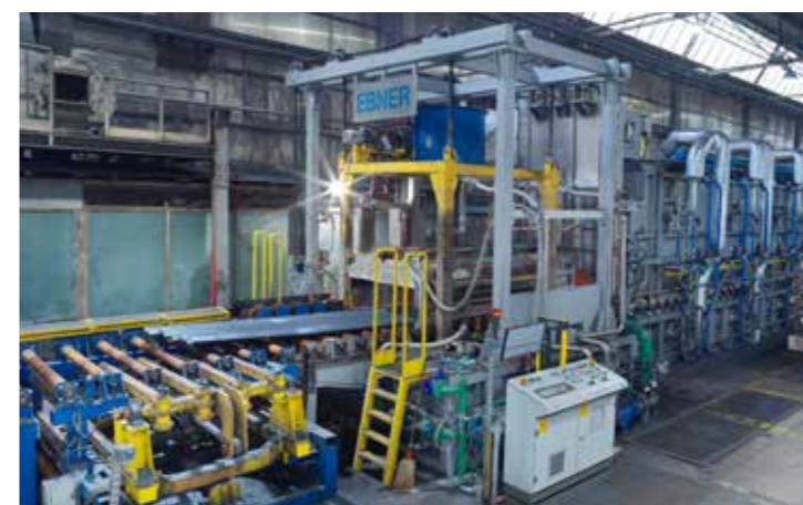
Quenching vessel for coils
